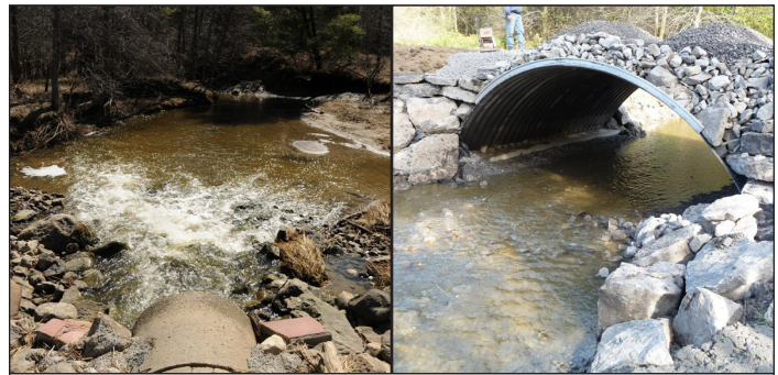
Figure 2. Original pipe culvert (left) that was replaced in 2010 with a bottomless arch culvert (right) in order to facilitate fish passage for migrant fish species from the St. Lawrence River.
